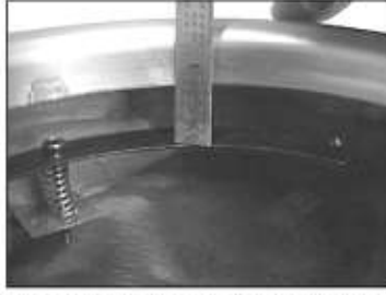
If you are using sealed beams adjust the lamp base to 1" from the trim ring I.D. If you are installing Hagan Blue Dot or Snake Eye lamps adjust base to 3/4".
